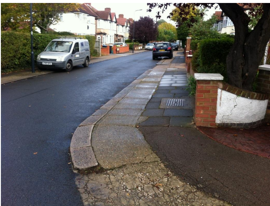
Medway Gardens: significant deterioration of concrete verges and crossovers can be seen
