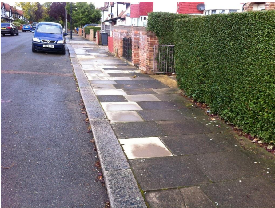
Medway Gardens - Original dark coloured slab paving is still exists, with lighter newer slabs being evidence of where repairs have had to be carried out
