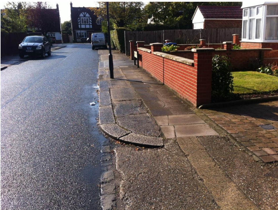
Medway Gardens: significant deterioration of concrete verges and crossovers can be seen
